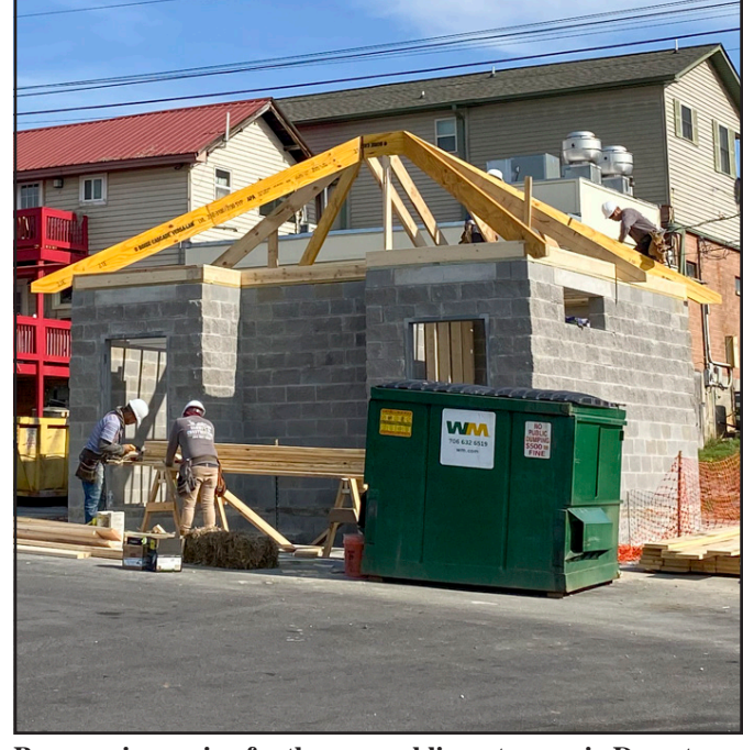
Progress is ongoing for the new public restrooms in Downtown Blairville, pictured here on Thursday, March 16.
